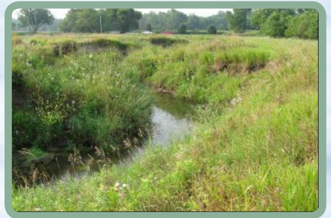
Figure 3. Bank instability in a ditch.
