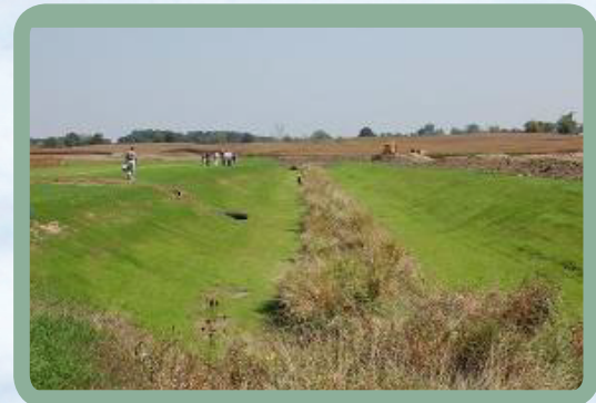
Figure 8. Construction of a two-stage ditch. The benches were made wide enough for vehicle access (top) and are located just below subsurface drainage outlets (above). Discharge from the outlets flows across vegetated benches.
