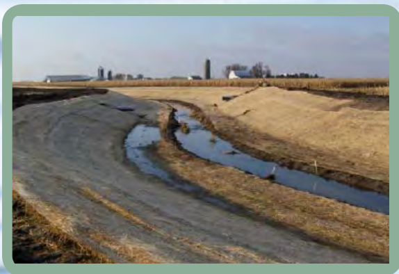
Figure 12. Geotextile fabric can be used to stabilize benches and banks until vegetation can establish.
