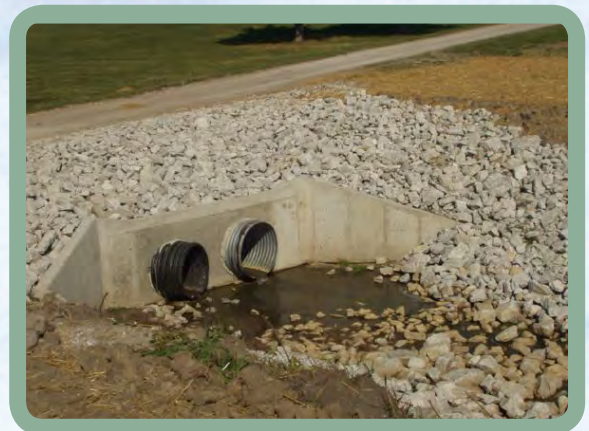
Figure 10. Rip rap can help stabilize stream banks, especially in transition areas. (source: http://seeversfarmdrainage.com )
