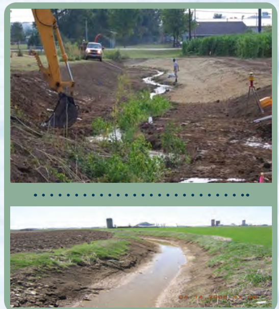
Figure 1. A. (top): construction of a two-stage channel. B. (bottom): traditional maintenance of a trapezoidal channel.
